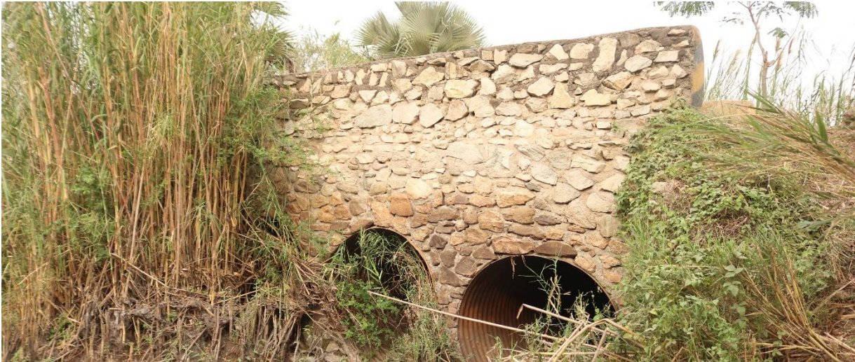
Plate 4-1: Status of the existing Road (Photos taken on 25th January 2025)
