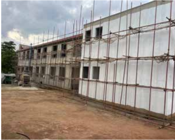
Fig (a): New Office Block under construction at the Central materials laboratory
