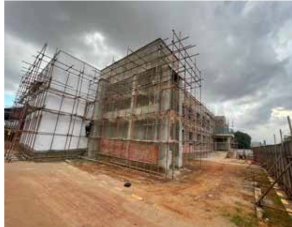
Fig. (b) new office block under construction at the Central material laboratory
